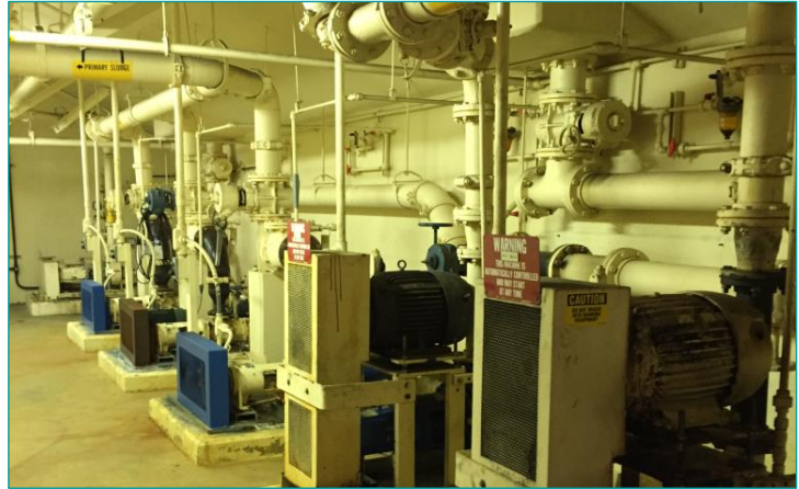
Pipe gallery, primary sludge pumps, and grit pumps.
