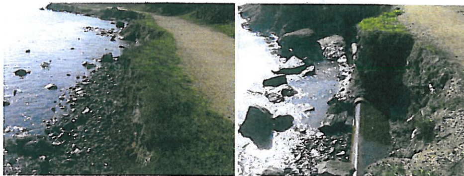
Figure 2. Ground photos of eroded bluff (looking south)
